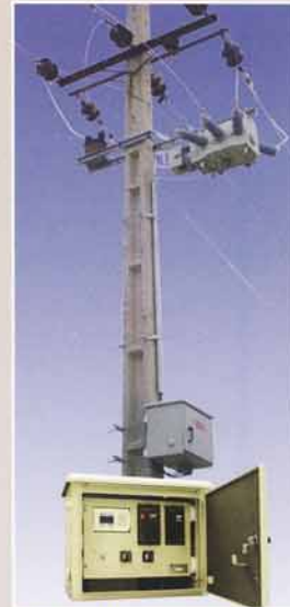
PGLM (RTU controlled)
